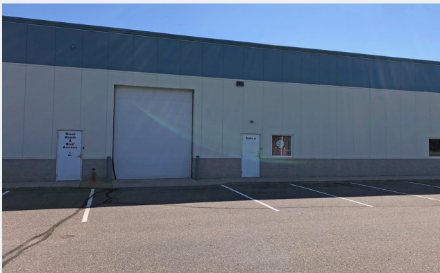
Drive in door
